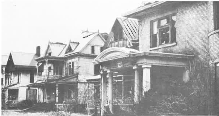
Deteriorated housing conditions, especially along the major arteries, is a problem for the community.
